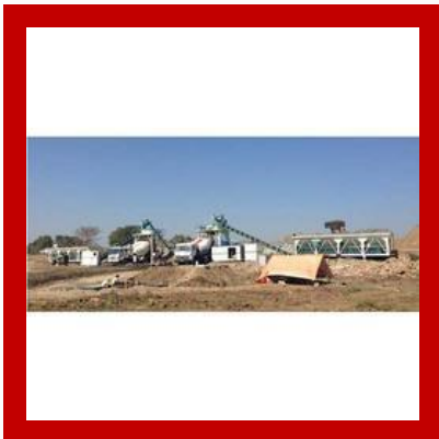
Pan Type Mobile Concrete Batching Plant
